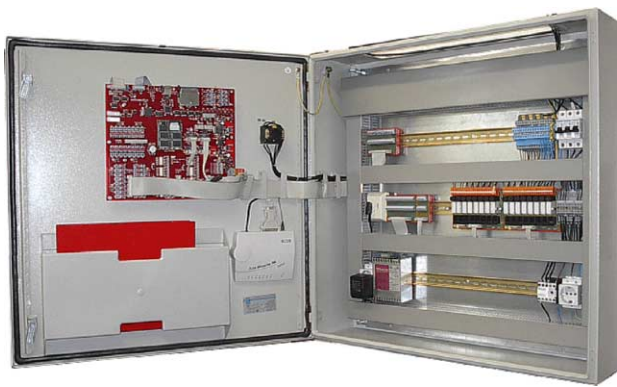
Fig. 2. Implemented microcontroller solution with input/output and switching modules [Foto: energiekontor Hannover].
